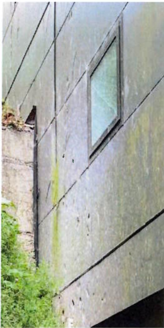
Figure 6: Damage to the Building
